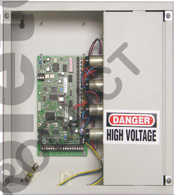
L28 interior displayed with cover removed and High Voltage cover in place.
